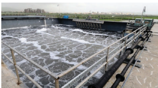
Figure 22.4 A view of sewage treatment plant
